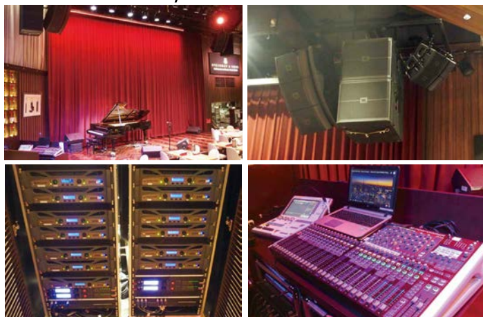
Mixing console, speaker system, power amplifier
